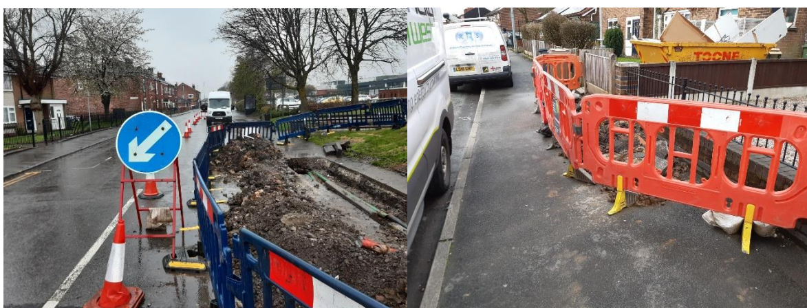
Figure 4: Photos of example ENWL roadside work sites. One (left) has an excavation across most of the footpath with spoil deposited on one lane of the road. The other (right) is constrained to half the width of the footpath. Both are exposed to the elements, with minimal space between barriers, excavation, and spoil.
