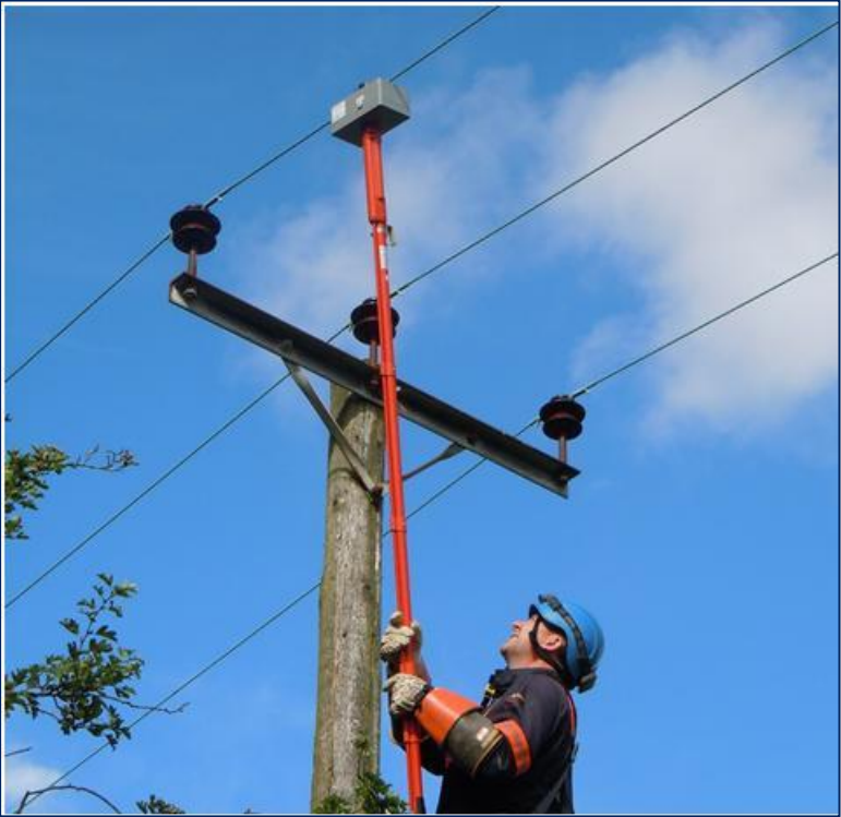
Figure 1: Dead-line installation of voltage logger device (used as part of earth fault detection algorithm development)
