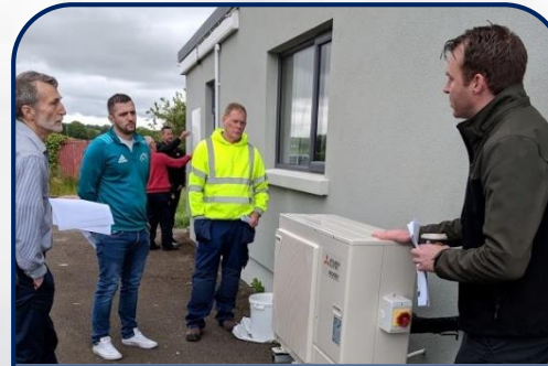
Carbon Coop Community Energy – Heat pump ready!
