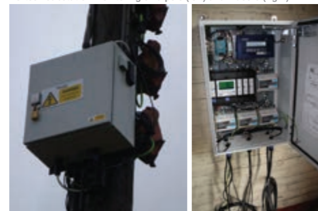
Nortech substation monitoring on a pole (left) and indoors (right)
