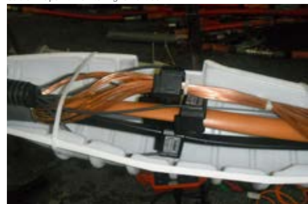
Cable midpoint monitoring 'Smart Joint'
